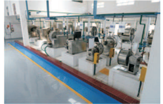
A view of equipment at the newly opened Clariant's Leather Excellence Centre
